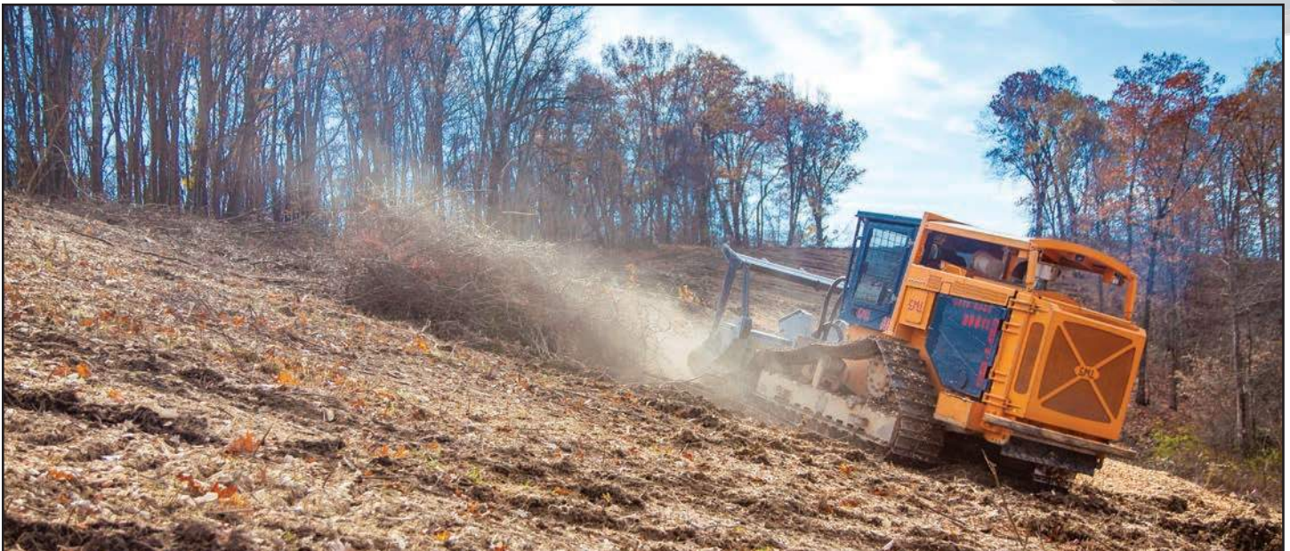
North Suburban Tree's CMI C450 mulcher—pictured clearing land around Range Resources' John Elliott 11826 well in Canonsburg, PA—needs to be "tough, well-engineered and safe", as Blum described, to handle unforgiving environments that can encompass 1,000 acres.
